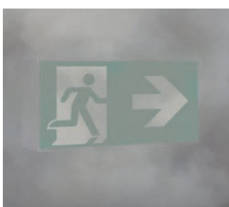
Badly illuminated escape sign
